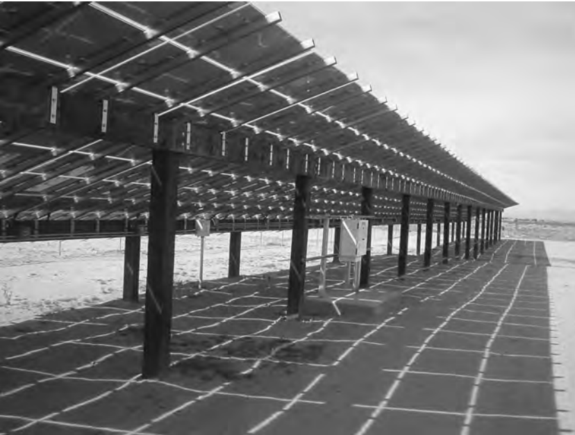
Figure B.24 Solar power farm installation in Mojave Desert. Photo courtesy of Grant Electric.
