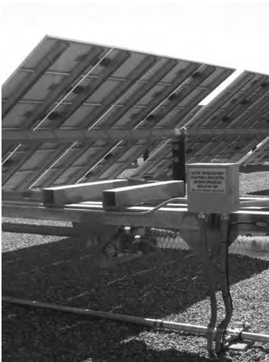
Figure 5.20 Solar tracking tilt actuator mechanism, Semitropic Water District, Wasco, California. Photo courtesy of Vector Delta Design Group.
