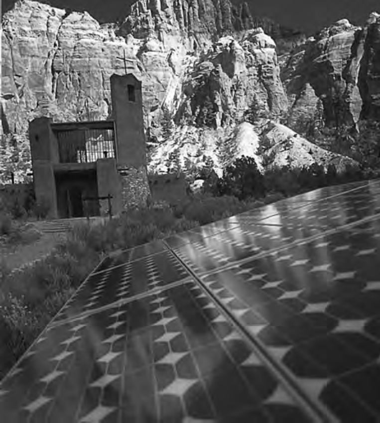
Figure B.18 Desert floor mount solar power installation.
