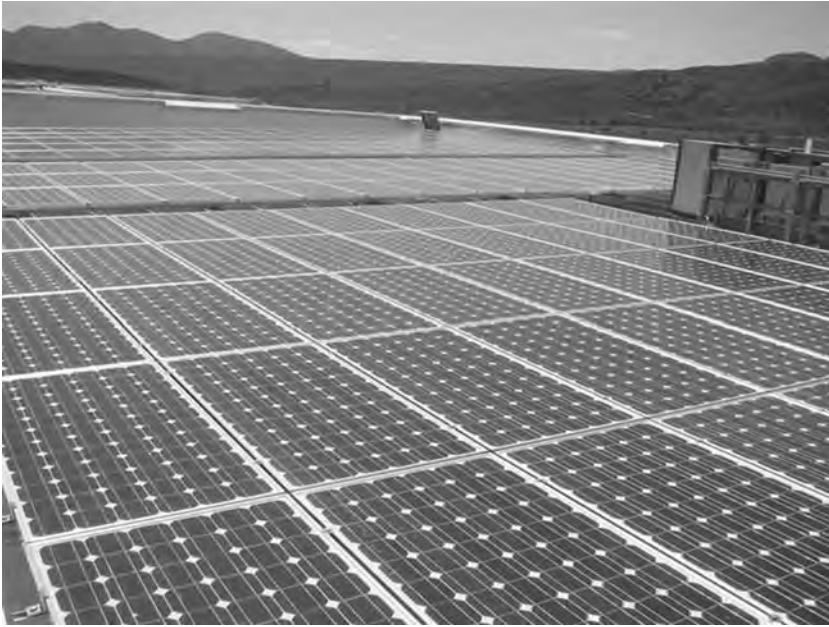
Figure 5.9 Water and Life Museum, rooftop solar power systems.
