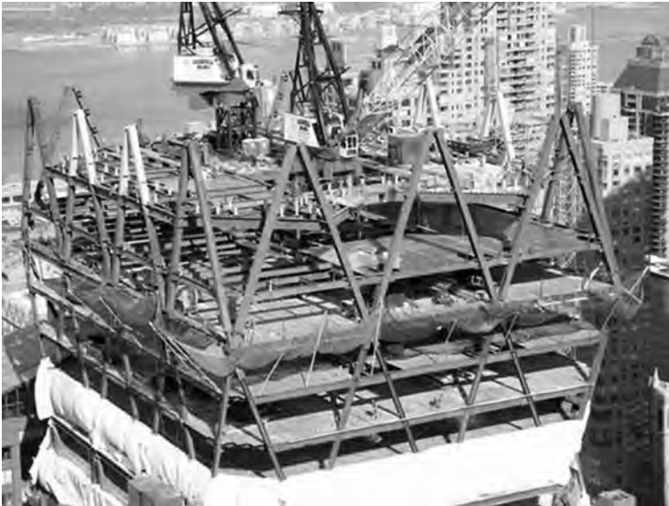
Figure 7.13 Digital structural members of new Hearst tower, New York, NY. Photo courtesy of Hearst Corporation.
