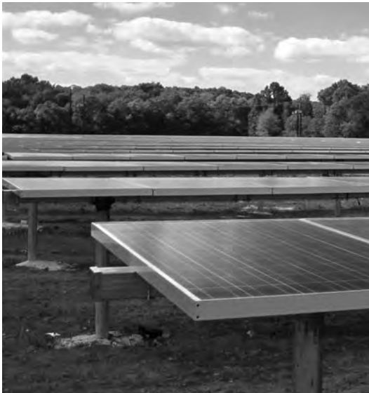
Figure B.35 Close-up of ground-mount single axis tracker solar power system. Photo
