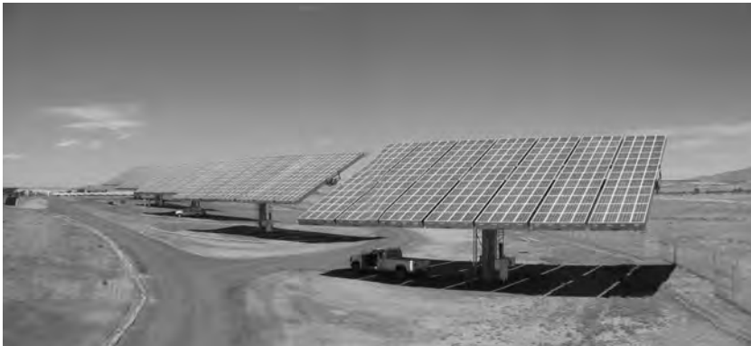
Figure B.22 30 KW Solar mega concentrator power co-generation farm. Photo courtesy of AMONIX.
