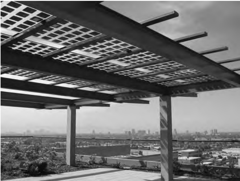
Figure B.30 BIPV solar power canopy installation. Photo courtesy of Atlantis Energy Systems.
