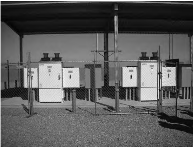
Figure 5.21 Solar power inverter installation, Semitropic Water District, Wasco, California. Photo courtesy of Vector Delta Design Group.
