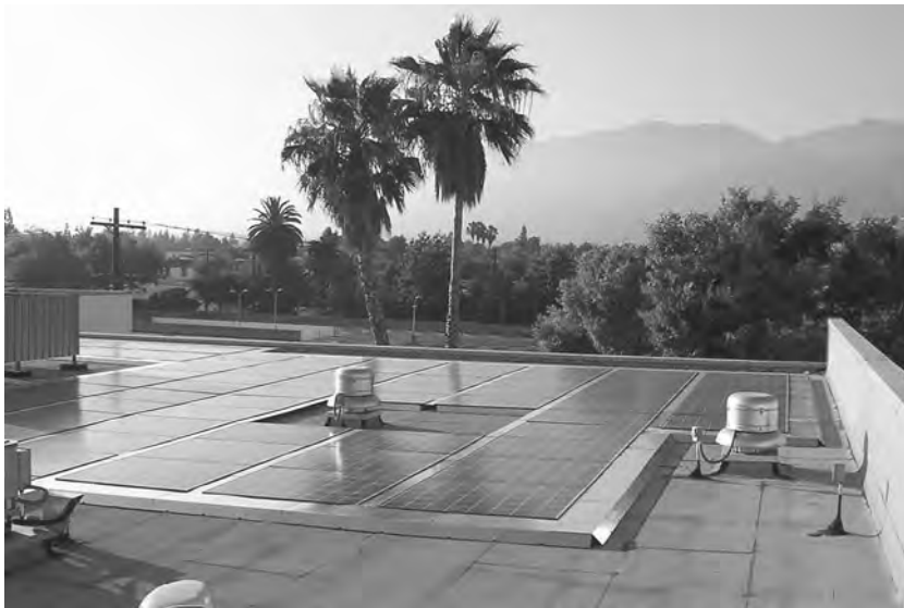
Figure 7.4 TriCom roof-mounted solar power cogeneration system.
