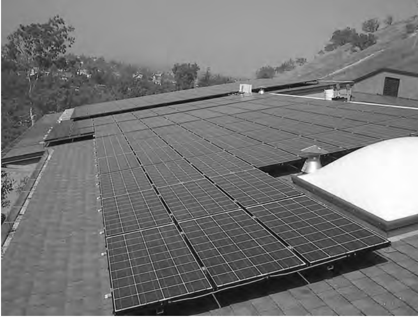
Figure 7.2 Los Angeles Audubon Center grid-independent solar power generation, system. Photograph courtesy of LA Audubon Society.
