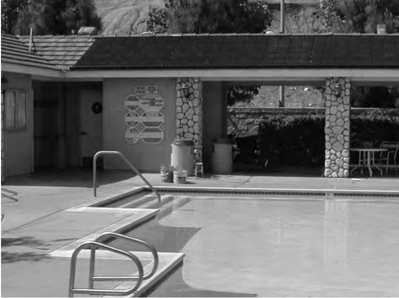
Figure 10.7 Residential roof-mount solar pool heater.
