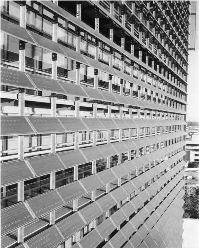
Figure 2.18 Application of BIPV as window canopy in CalTrans building, Los Angeles, California. Photo courtesy of Atlantis Energy Systems.
