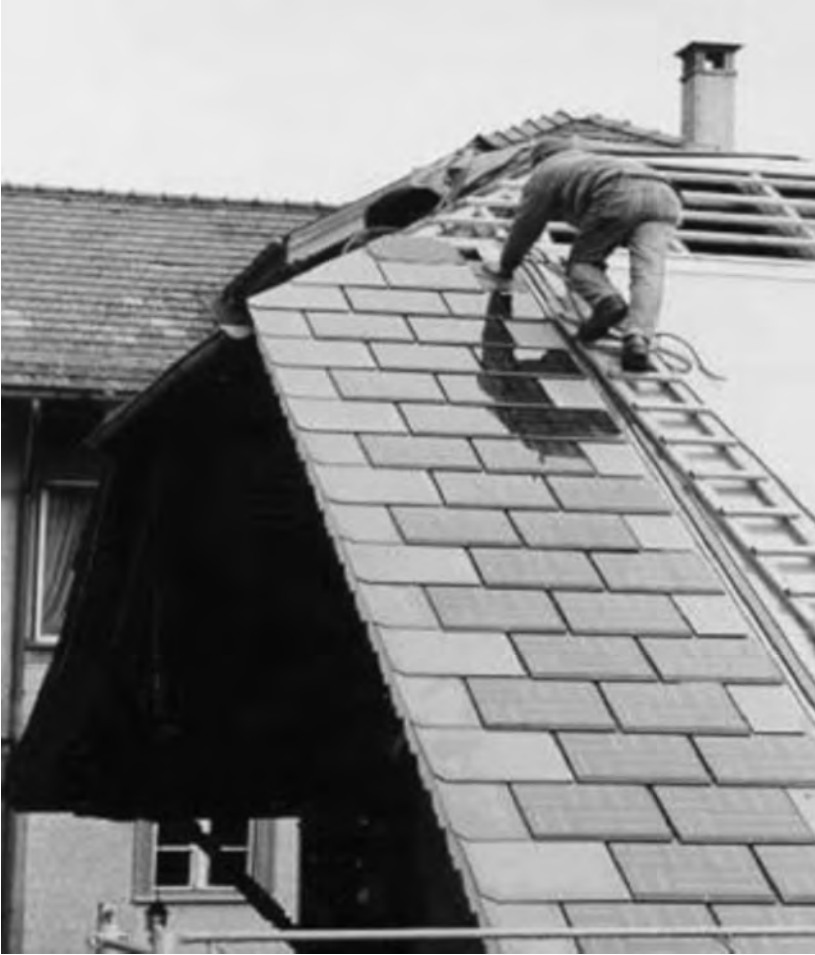
Figure B.26 Solar power roof slate installation in residential building roof structure. Photo courtesy of Atlantis Energy Systems.
