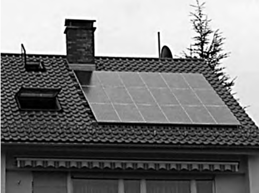
Figure B.27 Laminated glass solar power installation in residential building roof structure. Photo courtesy of Atlantis Energy Systems.
