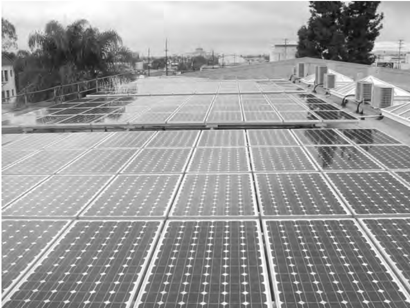
Figure 5.5 Roof-mount solar power system, Arshag Dickranian School, Hollywood, California. Photo courtesy of Vector Delta Design Group, Inc.
