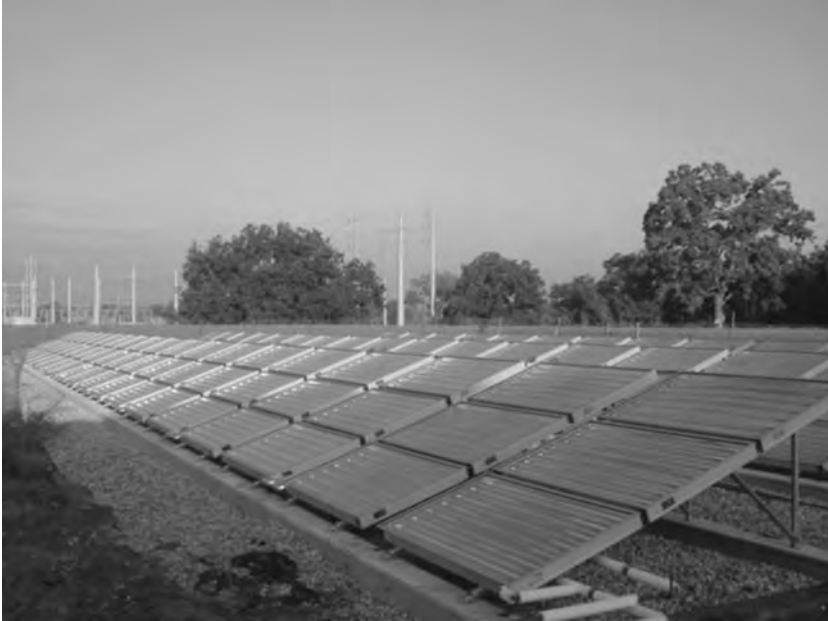
Figure 10.11 Parabolic solar heating system installation.
