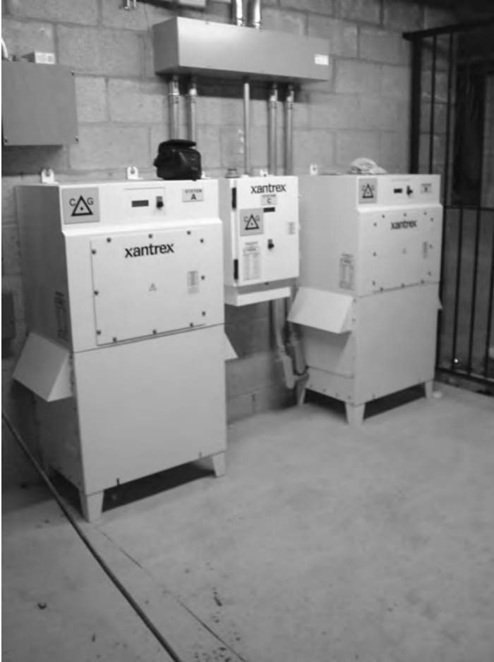
Figure 5.6 Inverter system, Arshag Dickranian School, Hollywood, California. Photo courtesy of Vector Delta Design Group, Inc.
