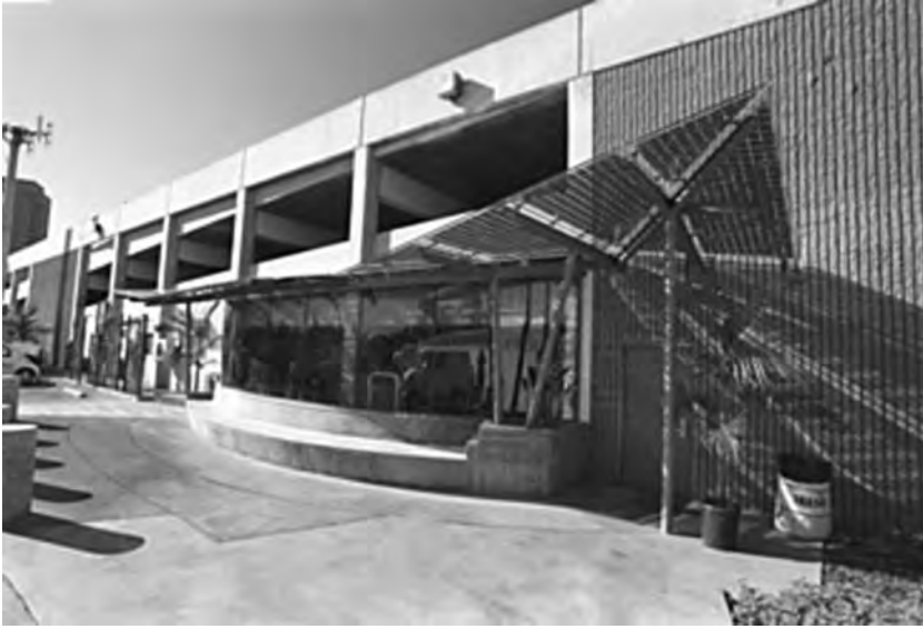
Figure B.29 Laminated glass BIPV solar power installation in commercial building entrance. Photo courtesy of Golden Solar Energy.
