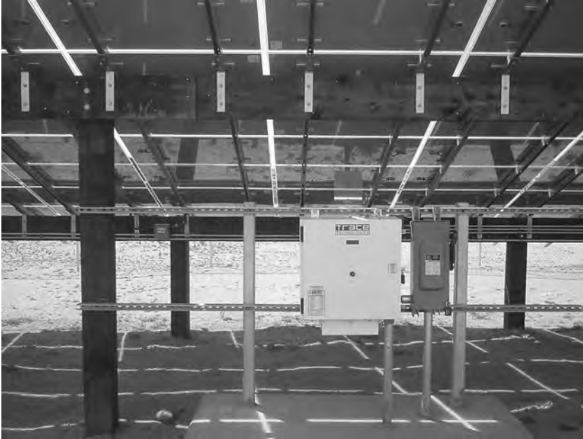
Figure 5.8 Boron solar farm inverter system. Photo courtesy of Grant Electric.
